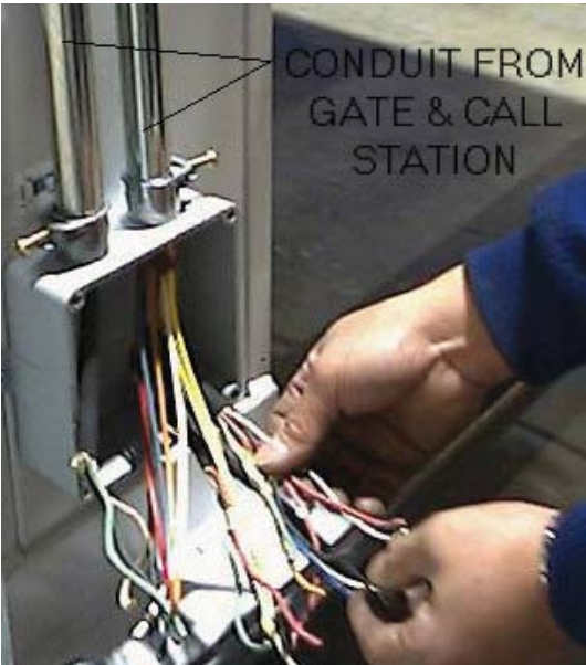
FIG. 18- WIRING OUTSIDE JUNCTION BOX
